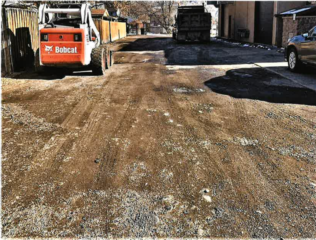
(Before, most of potholes are hard to see.)
