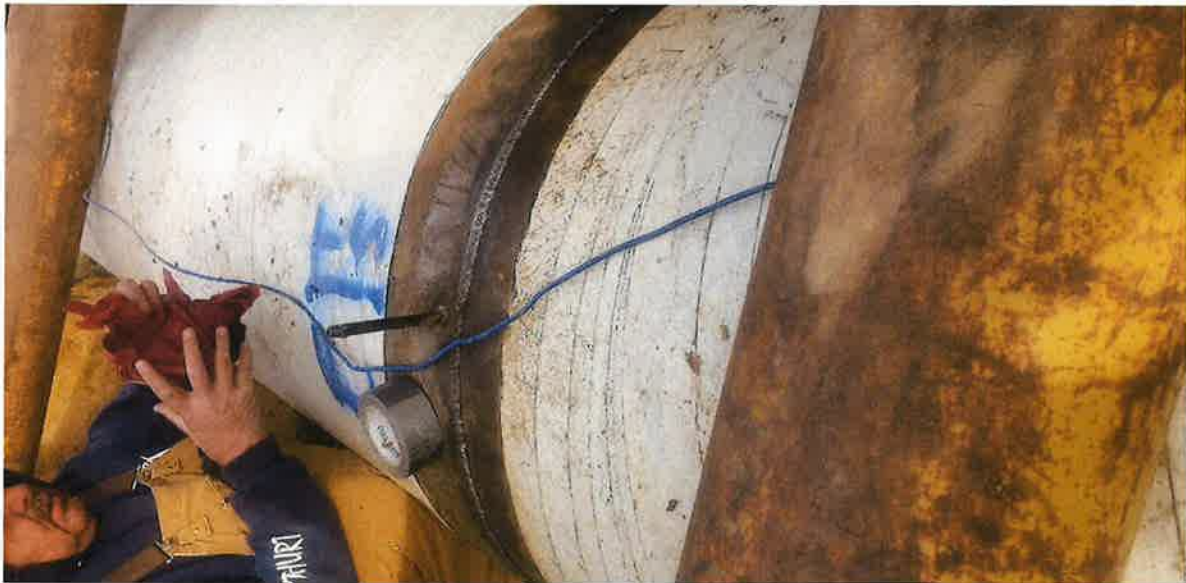
(You can see the weld along with a small pipe. After pipe is welded inside and out, they pressure test the joints for 5 min. If it fails, they grind the entire weld and start over.)
